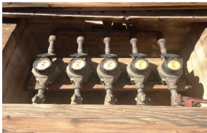
Figure 2. Shared well metered service connections with shutoff valves. Source: G. Hix.
