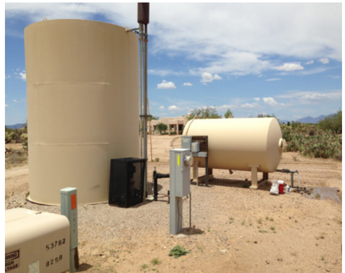
Figure 1. Shared Well storage and pressure tanks. Source: G. Hix.
