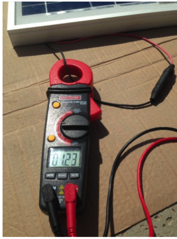
Figure 10. Measuring short-circuit current ( I_{sc} ) with a clamp-on DC multimeter to check if the rated short-circuit current ( I_{sc} ) value matches the specification sheet.
