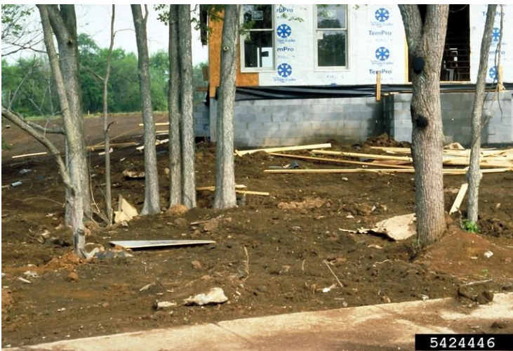
Construction activity has buried the bases of these trees which often leads to butt rot and tree mortality (John Hartman, University of Kentucky, Bugwood.org).
