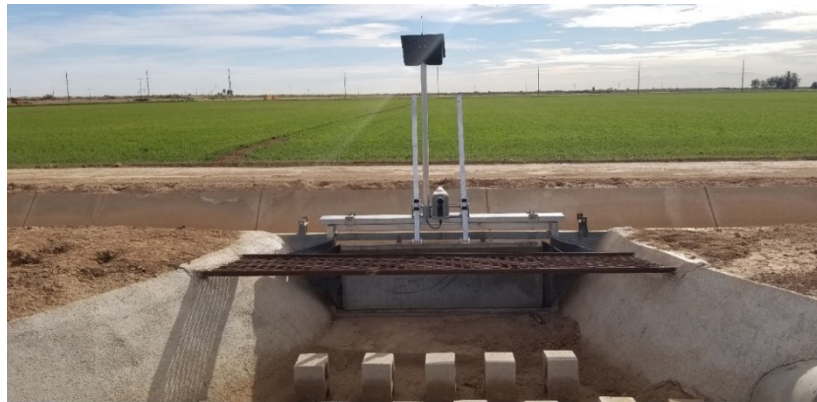
Figure 3. An automated bay outlet for border check surface irrigation. (Credit: Rubicon Water. Used by permission)
