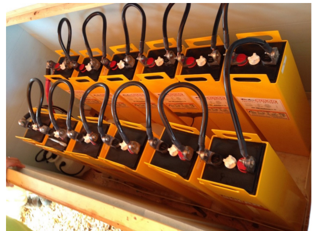
Figure 14. Example of 20 2-volt batteries wired in series produce a 24-volt battery bank. The positive terminal of each battery is connected to the negative terminal of the next battery. Source: Author.
