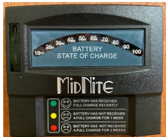
Figure 25. Battery monitor is used to show state of charge of battery bank. Source: Author.
