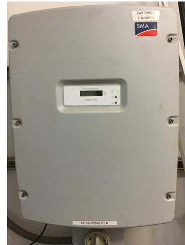
Figure 24. A larger system inverter for off-grid systems. This unit is part of a system at an off-grid charter school in Northern Arizona. Source: Author.
