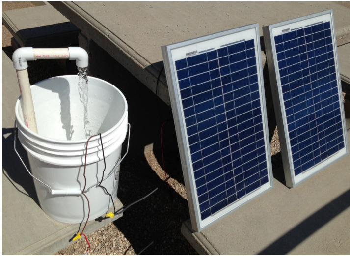
Figure 4. Two 17-volt modules wired in series produces 34-volts of electricity to increase the electrical power to the DC load. Source: Author
