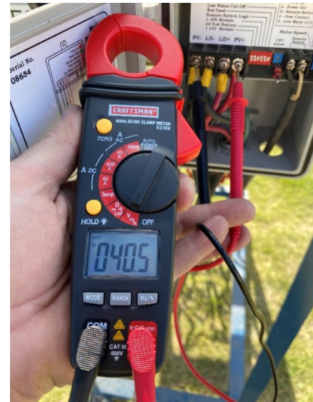
Figure 24. Taking a voltage reading of the PV with the digital multimeter Source: Author
