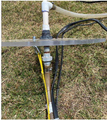
Figure 12. Acrylic lid with pipe fittings attached. Source: Author
