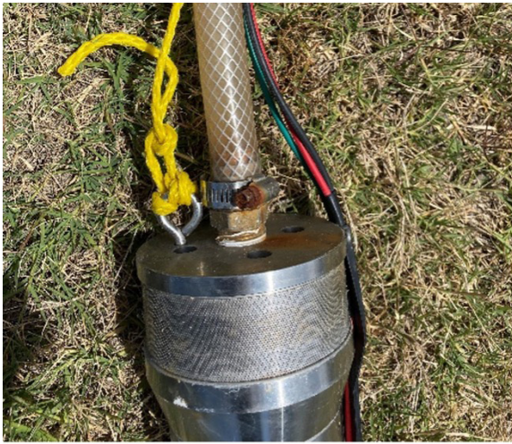
Figure 17. Eyehook installed in top of pump with safety rope attached.
