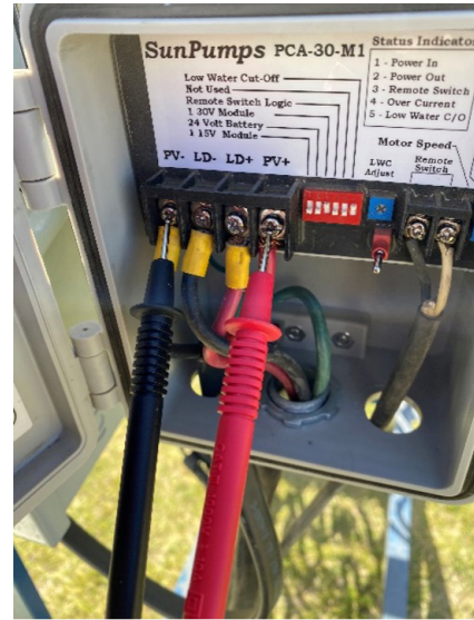
Figure 23. Checking the voltage on the PV connections of the pump controller with the digital multimeter. Source: Author
