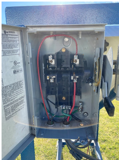
Figure 5. Safety disconnect switch is a recommended feature. Source: Author
