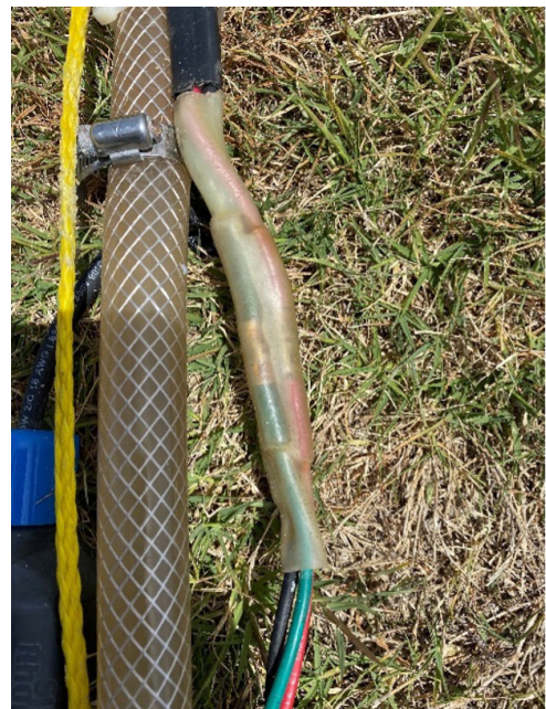
Figure 16. Wires from pump are spliced and sealed with silicon to prevent corrosion.
