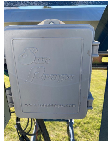
Figure 6. Solar pump controller Source: Author
