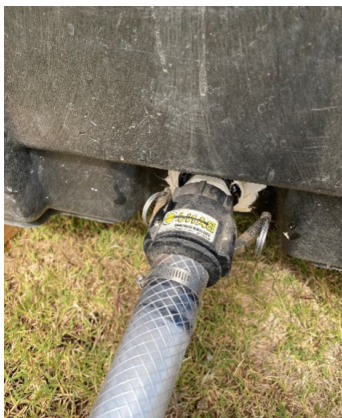
Figure 19. Stock water trough with a banjo connector fitting. Source: Author
