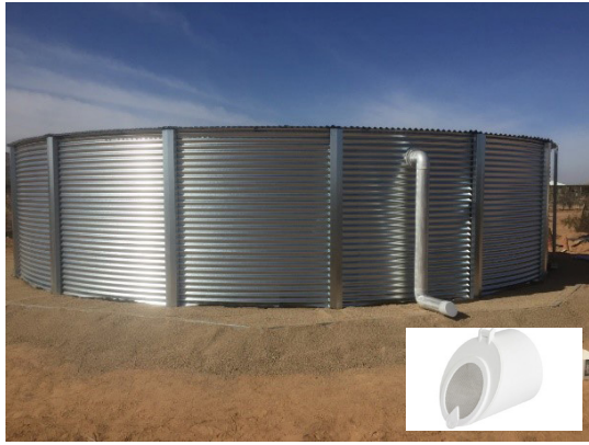
Figure 7. Top: White overflow pipe comes out of large steel tank. Photo courtesy of Oasis Water Harvesting. Insert: Mozy flap valve screen keeps out critters and mosquitoes. Photo courtesy of the Blue Mountain Company.
