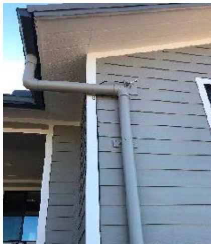
Figure 2. Large diameter downspout pipes keep water flowing smoothly.
