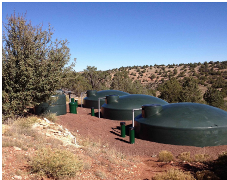
Figure 8. A 300-gallon tank, on the left, serves as a settling tank before water goes to three linked 5,000-gallon tanks. Photo courtesy of Thad Johnson.
