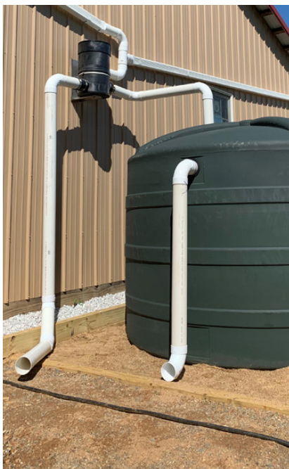
Figure 4. WISY Vortex fine filter roof washer attached to two downspouts. The vertical pipe on the left is outflow for 'debris' water discharged by the unit at about 90% water efficiency. Photo courtesy of Rainwater Management Solutions.
