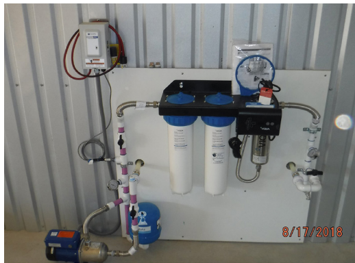
Figure 14. Left: A rainwater installation with an on-demand pump, a 10-micron sediment filter, a 5-micron activated carbon filter, and a UV lamp. Photo courtesy of Chris Maxwell-Gaines.
