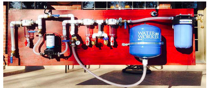
Figure 16. Following a pump and two spin-down filters, a 6-candle ceramic filter (far right) is the last component in this Aqua AXIS rainwater purification system. Photo courtesy of Neal Gist, Ozark Permaculture LLC.
