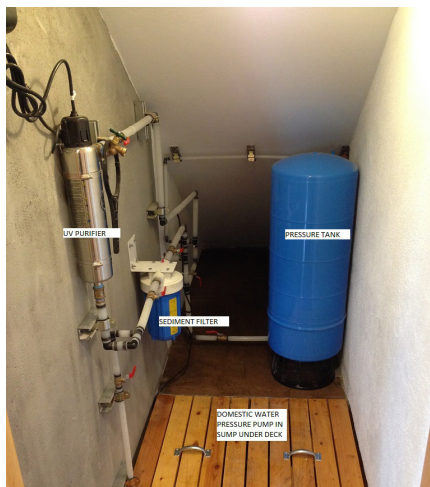
Figure 15. Right: Due to purity of the captured rain in this system, one sediment filter and a UV lamp are all that is needed. A Grundfos MQ 3-45 on-demand pump, under the floor, is coupled with a pressure tank to reduce the pump's on/off cycles. Photo courtesy of Thad Johnson.
