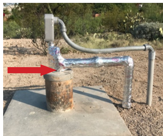
Figure 2. Arrow points to an opening a well seal where all sounder readings can be referenced. Source: G. Hix
