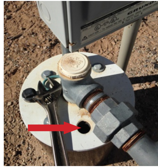
Figure 6. Arrow points to access port in a well seal where a sounding tube could be installed. Source: G. Hix
