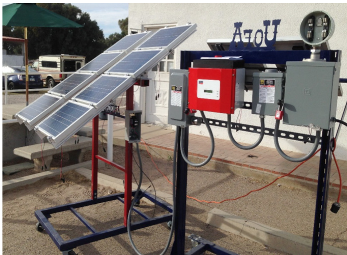
Figure 1. A grid-tied system is used to produce energy for the user during the day, sends excess energy to the local utility, and relies on the utility to provide energy at night. The system pictured is a small-scale PV demonstration featuring all of the components: a PV array and combiner box mounted on a racking system, a DC disconnect switch, a string inverter (red and white unit), an AC disconnect switch, and an AC service panel. Collectively, these are referred to as the Balance of System (BOS).
