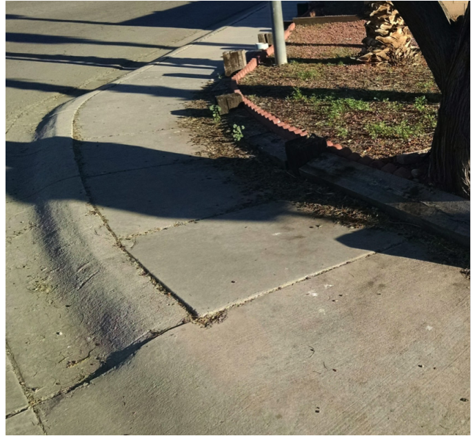
Figure 6. The roots of large and aggressive trees occasionally cause damage as they grow underneath sidewalks, pavement, and foundations. Choosing the right tree for these locations coupled with good soil preparation are key steps in avoiding structural problems.
