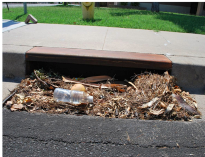
Figure 8. Storm Drain Clogged with Litter and Debris
