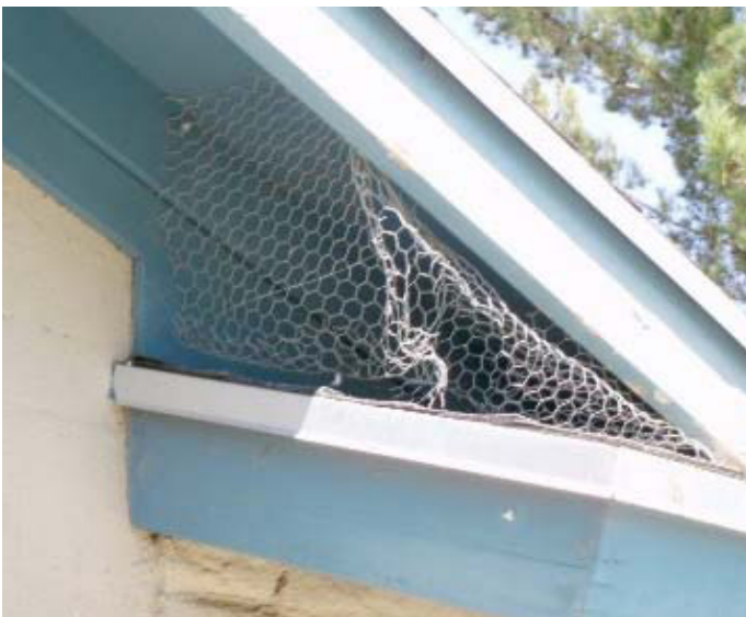
Fig. 18. Wire netting helps to keep birds and rodents out, but needs to be monitored and maintained.
