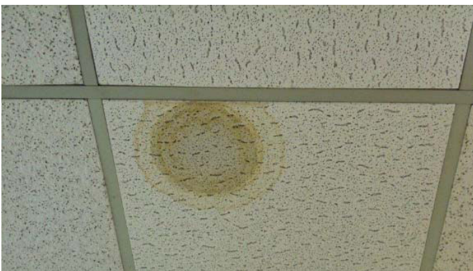
Fig. 8. Ceiling tiles indicating a roof or plumbing leak.
