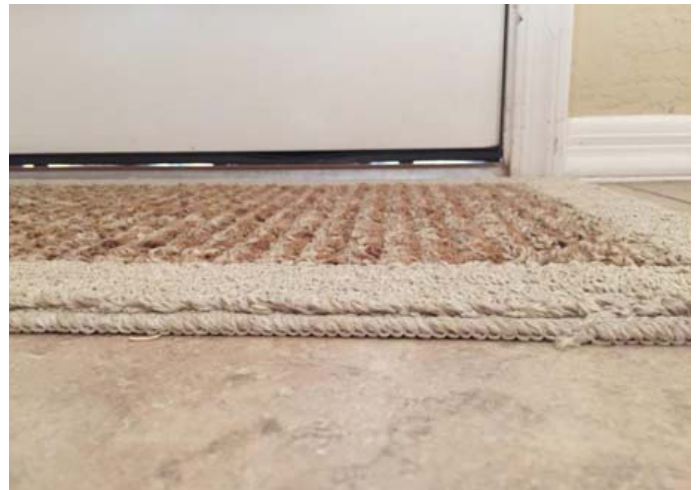
Fig. 1. This locked door is wide open to pests! (Note gaps under door).
