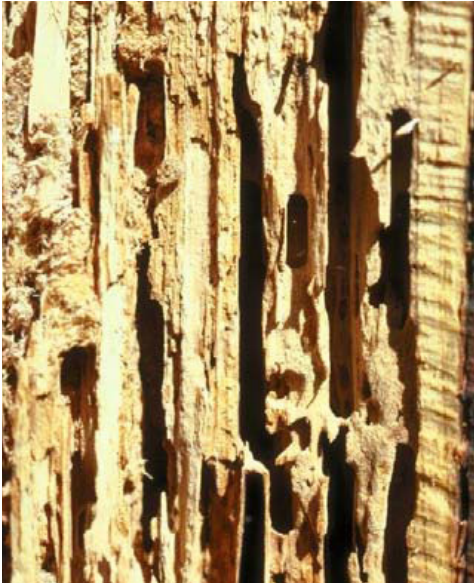
Fig. 24. Carpenter ant damage Photo: R. Werner, Bugwood.org
