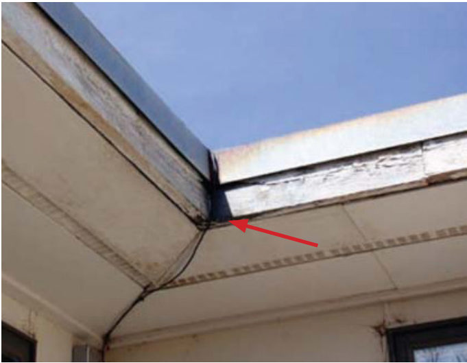
Fig. 17. Gaps under roofline can attract birds and rodents.
