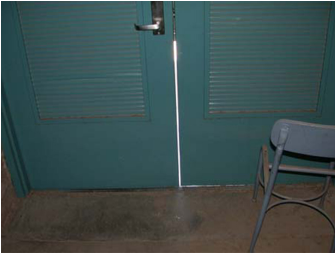
Fig. 3. Doors with worn-out door seals can be identified by light coming in through the gaps around the door.
