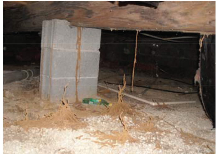
Fig. 45. Subterranean termite shelter tubes. Photo: Larry Ralph Jr., www.indiancrawlspacerepair.com .
