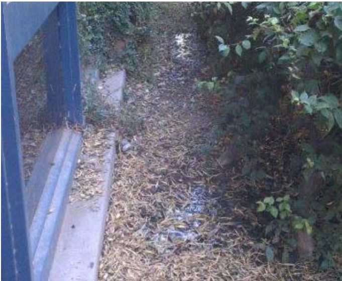
Fig. 13. Fallen leaves and other debris around the building provides harborage for pests and also holds moisture which can weaken the foundation.
