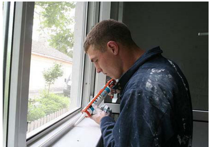
Fig. 6. Sealing cracks/gaps around window and door frames keeps pests out Photo: US Gov. Public Domain image.
