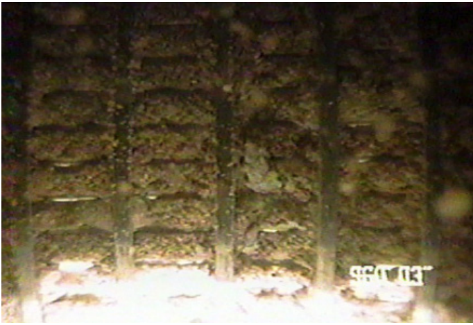
Figure 7. Wire wrapped well screen plugged with slime and mineral deposits. Photo by G. Hix.
