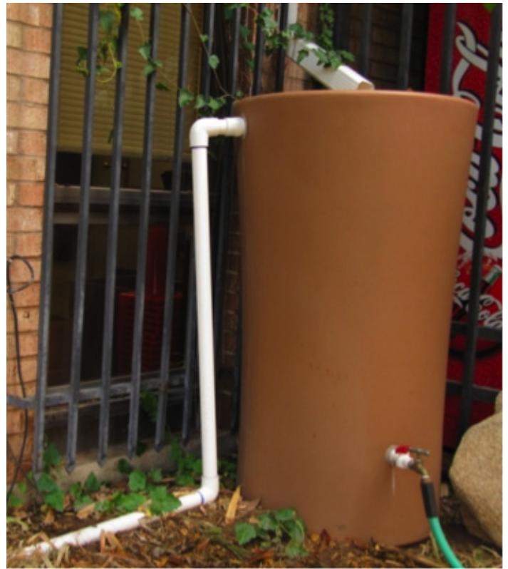
Figure 3. The overflow pipe—made with PVC (or ABS) material found at your local hardware store—takes water away from the cistern and the foundation of the building in the event that the cistern fills to capacity.
